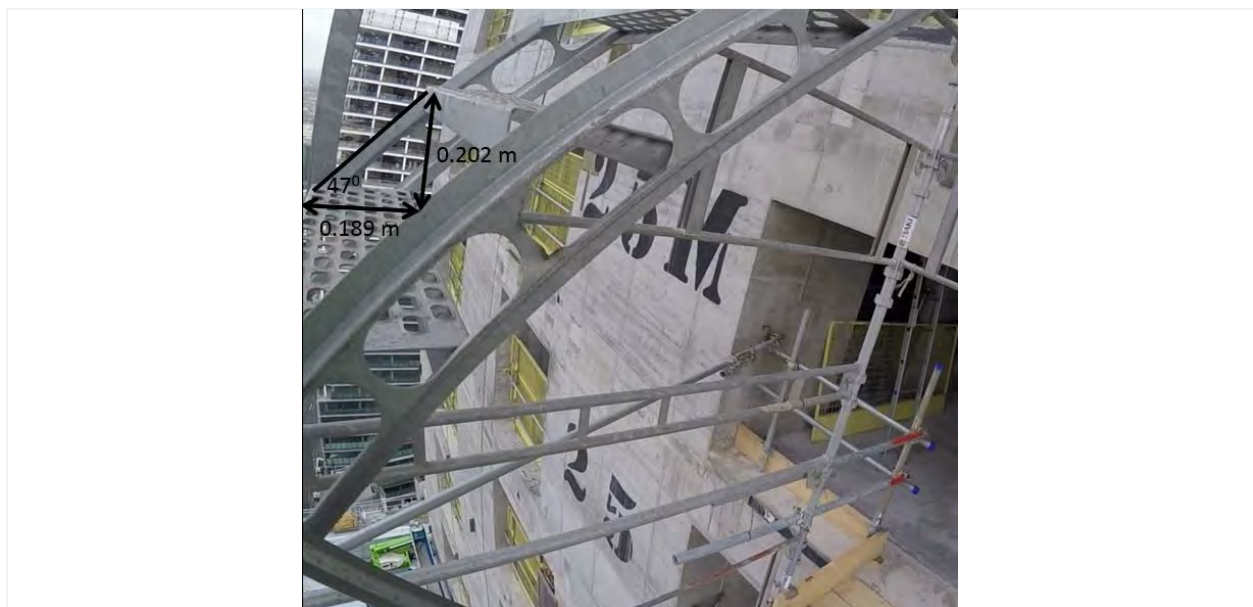
Figure 97. Tread and riser dimensions for the temporary scaffold dogleg stairs used in Trials 2 and 4.
