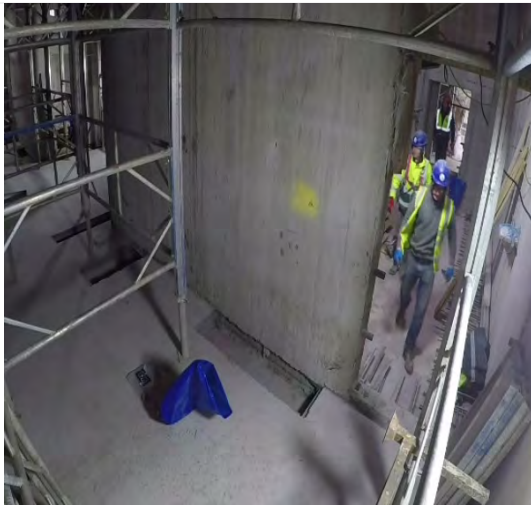
(a) MEP workers evacuating past other workers who are still engaged in work activities (out of view of the camera). A supervisor (in black with red helmet) is approaching the area.
