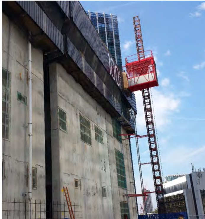
Figure 14. External hoist at 100 BG.
