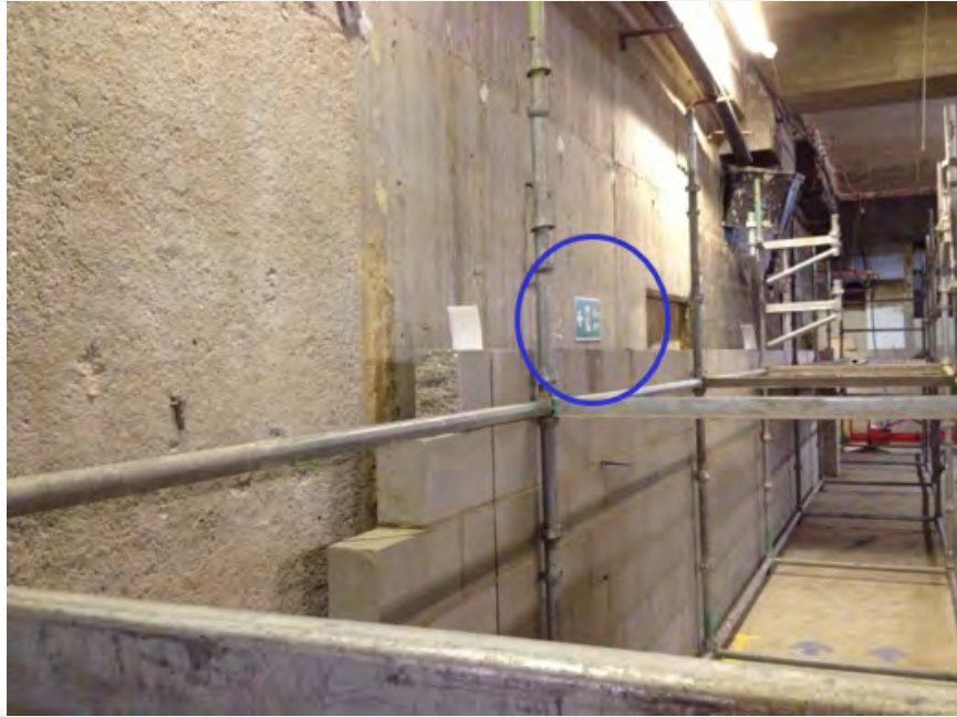
Figure 3. Emergency exit sign about to be obscured by work on the construction site.
