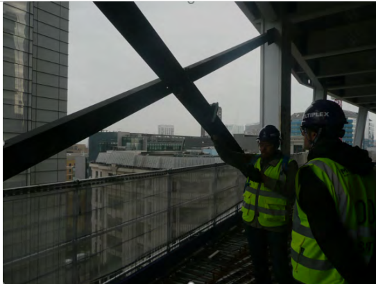
Camera (7) being set up on Level 7 on floor.
